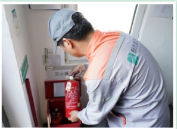
機房滅火器巡檢 Fire extinguisher inspection in equipment rooms
